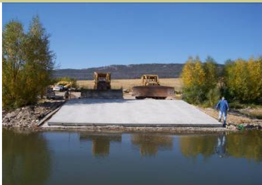
The slab for the new boat ramp weighed 50 tons but was pushed into place with hardly a ripple.
